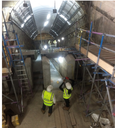
Viewing the escalators from Ticket Hall level
